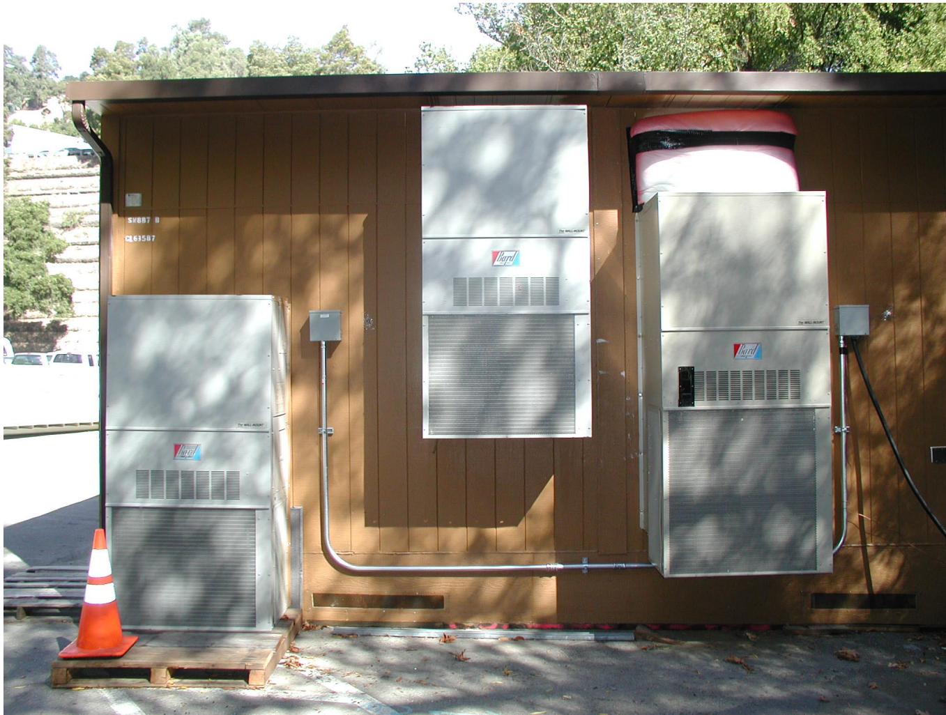
Figure 2. External wall of LBNL RC Test Bed showing the 10 SEER (left) and prototype IHPAC (right) wall-mount units. Batt insulation seen above the IHPAC was used prior to completion of an insulated top discharge duct. The third HVAC system on the far left was the original system on this RC.
