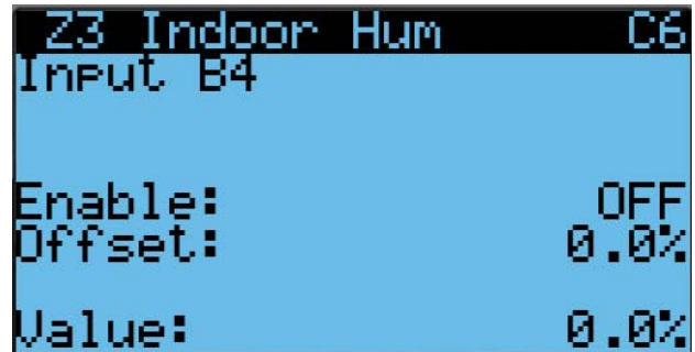
FIGURE 38 Enable/Disable Zone 3 Indoor Humidity Sensor
