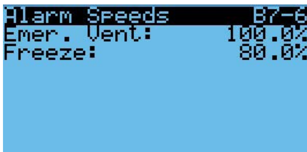
FIGURE 29 Adjusting Emergency Vent and Freeze Speeds
