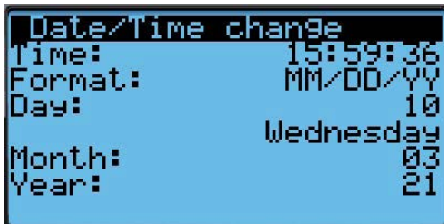
FIGURE 35 Setting Controller Date and Time
