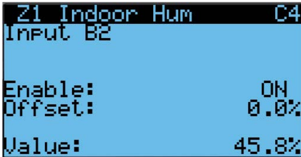
FIGURE 36 Enable/Disable Zone 1 Indoor Humidity Sensor
