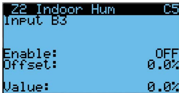
FIGURE 37 Enable/Disable Zone 2 Indoor Humidity Sensor
