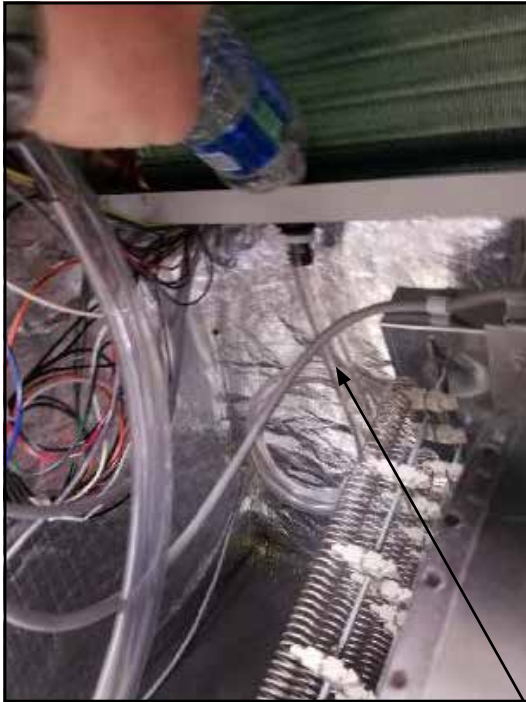
Evaporator Drain Pan Left Side Drain Hose
