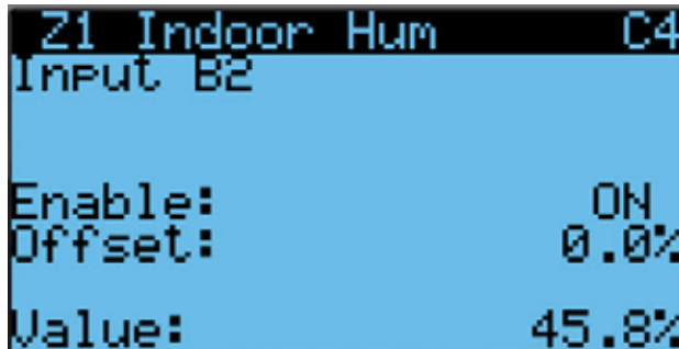
FIGURE 44 Enable/Disable Zone 1 Indoor Humidity Sensor
