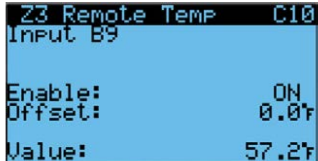
FIGURE 40 Enable/Disable Zone 3 Remote Temperature Sensor
