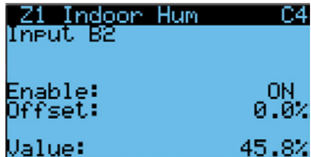
FIGURE 33 Enable/Disable Zone 1 Indoor Humidity Sensor
