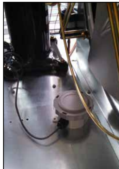
FIGURE 3 Outdoor Sensor Installation
