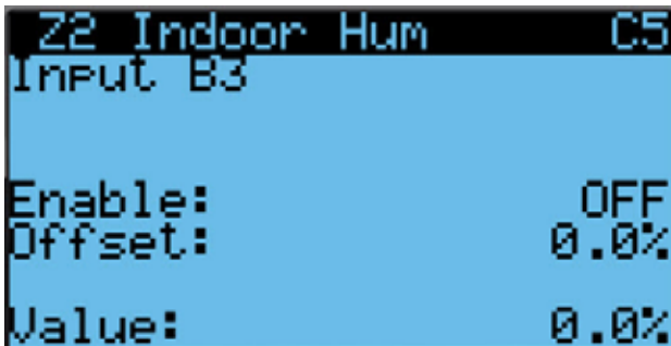
FIGURE 37 Enable/Disable Zone 2 Indoor Humidity Sensor
