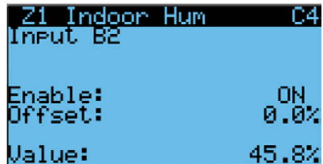
FIGURE 35 Enable/Disable Zone 1 Indoor Humidity Sensor
