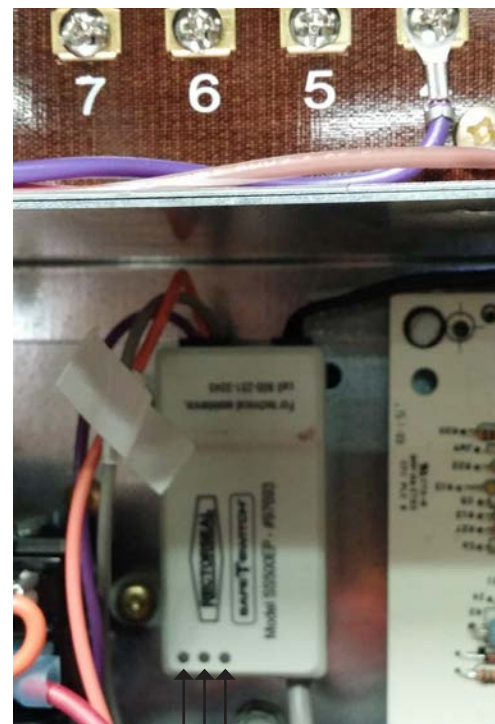
FIGURE 20 Outdoor Condensate Control
