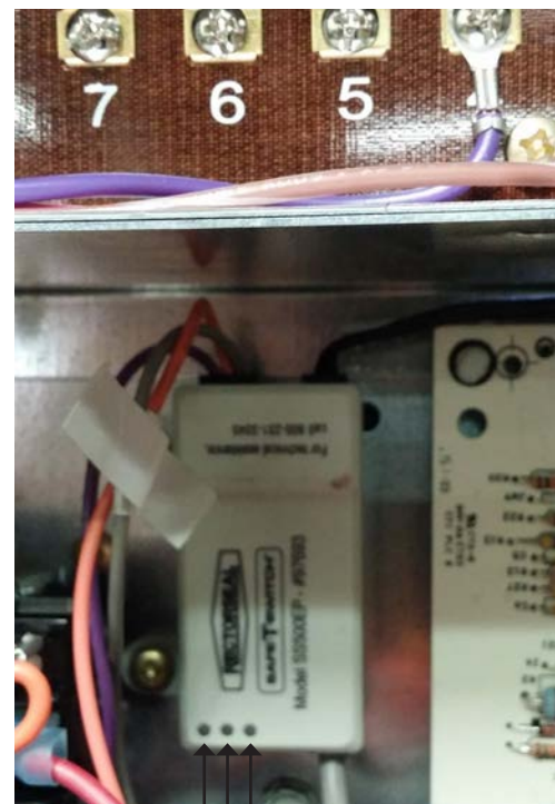
FIGURE 20 Outdoor Condensate Control
