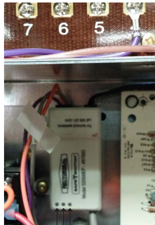
FIGURE 20 Outdoor Condensate Control
