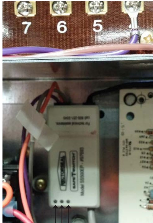
FIGURE 36 Outdoor Condensate Control
