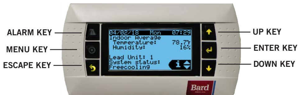
FIGURE 44 LV1000 Controller Display and Interface (Status Screen Shown)
