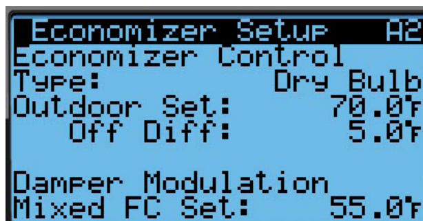
FIGURE 35 Changing Economizer Control Type
