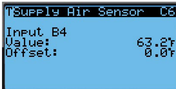
FIGURE 37 Supply Air Sensor
