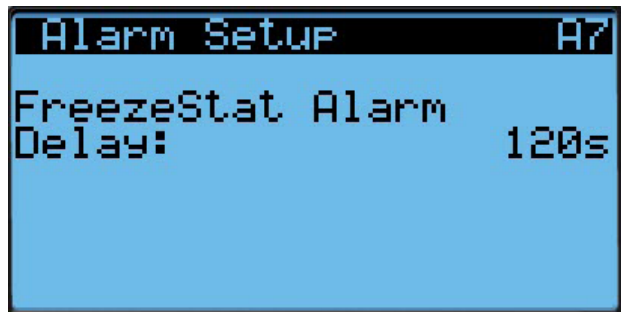
FIGURE 22 Adjusting Freezestat Alarm Delay
