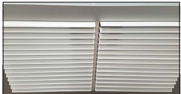
FIGURE 8 View of Installed Grille (as seen from above)
