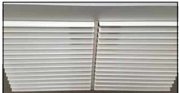
FIGURE 7 View of Installed Grille (as seen from above)
