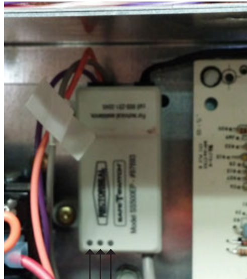
FIGURE 19 Outdoor Condensate Control
